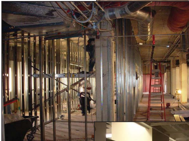
12/7/10 - (left) Metal framing is put up and the walls start to take shape.
